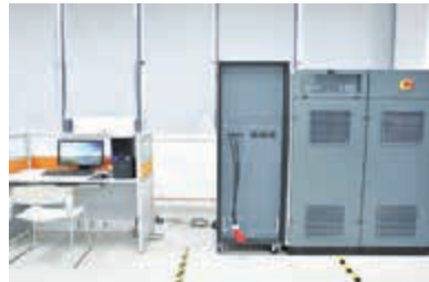
Harmonics & Flicker Test Laboratory
